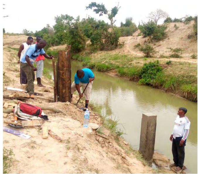
Kenya Water Resources Management Authority establishing water quality monitoring station on Mwache River
